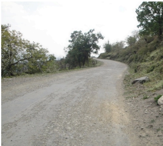
Pavement Failure due to insufficient cross drainage (Hakha-Gangow Road)
