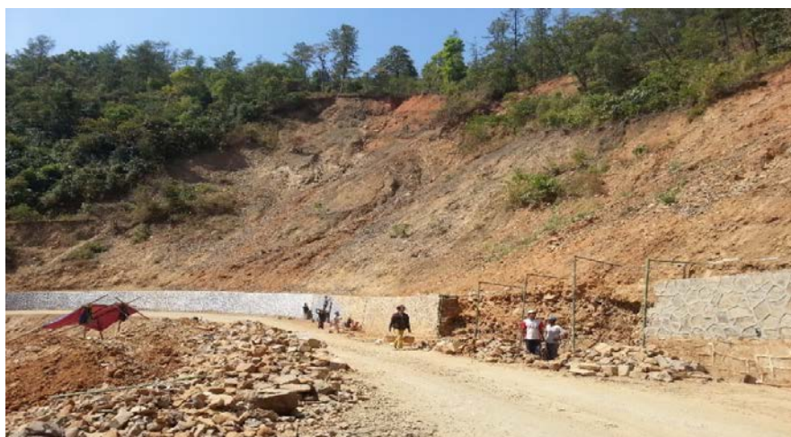
Retaining wall construction for landslide control. This retaining wall failed because additional drainage and other measures were not in place (Hakha- Gangaw Road)
