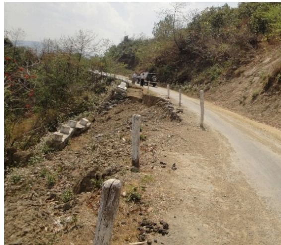
Retaining wall failure due to seepage and runoff of accumulated water (Kalay-Hakha Road)
