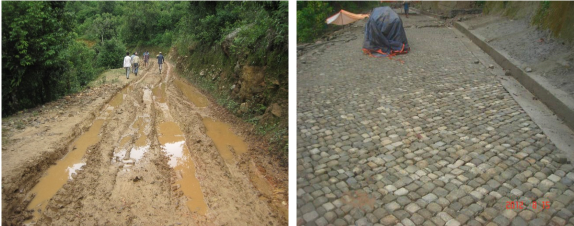
Photographs show the before and after situation of cobble road construction in Nepal
