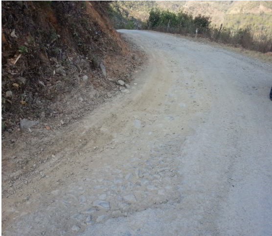
Paved Road with poor water management (Hakha - Gangaw Road)
